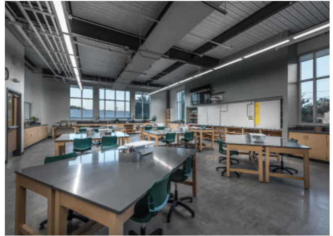
Classroom-lab with exposed mechanical system
