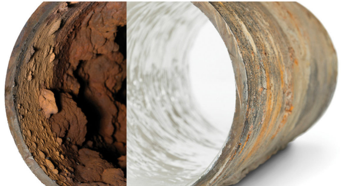
An Epoxy Brush Coating was applied in the pipes of the Vivarium's Cage Washing system to increase waterproofing, strength, and durability.
