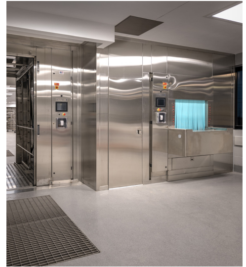
A 1' deep structural pit was inset to accumulate the run off from the vivarium's hydro-washer.
