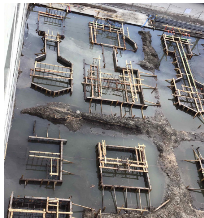
The site of the new central plant was flooded in July 2019, one of the many weather events that impacted the site.
