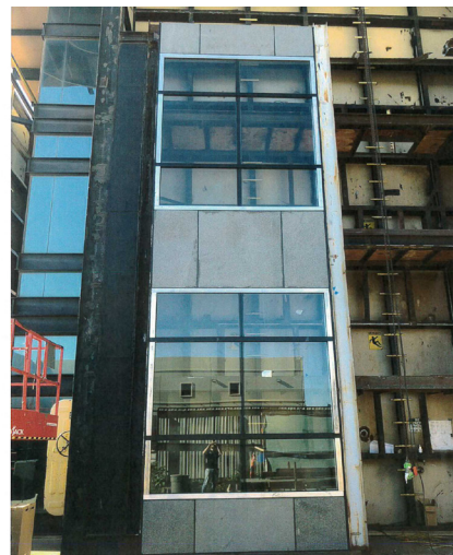
The exterior glass curtain wall system's performance was mocked-up and tested for wind and water penetration in Texas.
